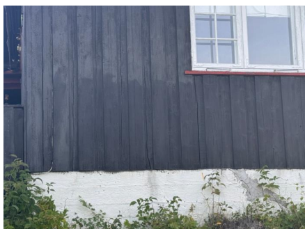
Sprekker i panelbord
