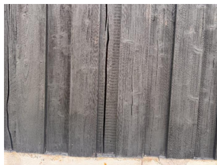
Sprekker i panelbord
