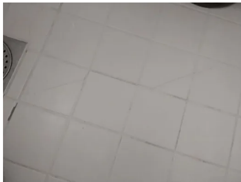
Sprekker i flis/fuger.
