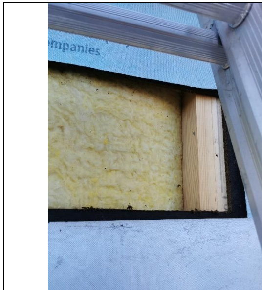
Mangelfull isolering, hulrom
