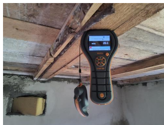
Overflate himling - Fuktmåling i himling.
