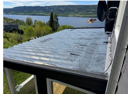
Slitt taktekking over veranda
