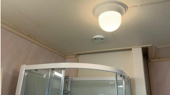
Noe fuktskjolder i himling
