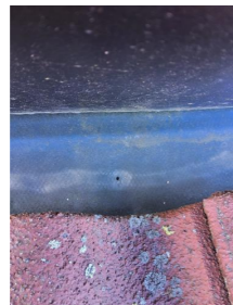
Skorsteiner (over tak) - Observert hull i tetting rundt pipe.
