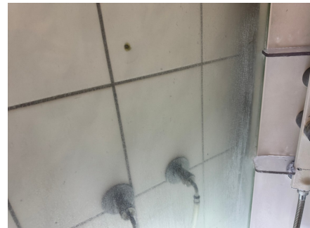
Hull i vegg bak kabinett
