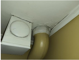
Overflater himling - Fuktskader i himling
