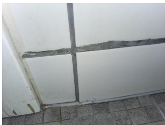
Overflater vegger - Riss/sprekker flisfuger
