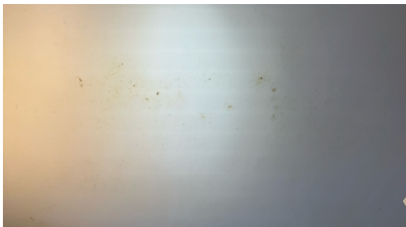
Misfarging i himling.
