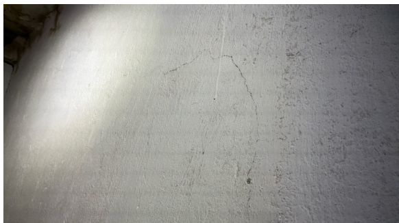
Sprekker/riss i pipe.
