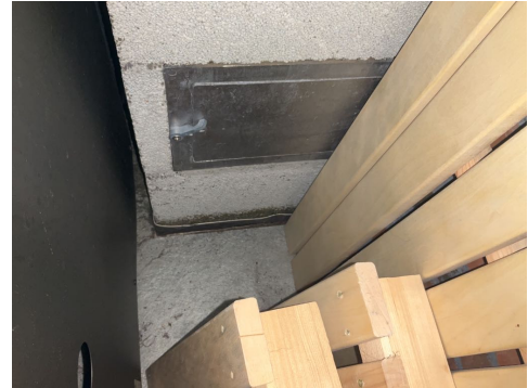
feieluke mangler ubrennbar plate under
