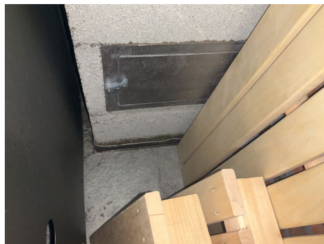
feieluke mangler ubrennbar plate under
