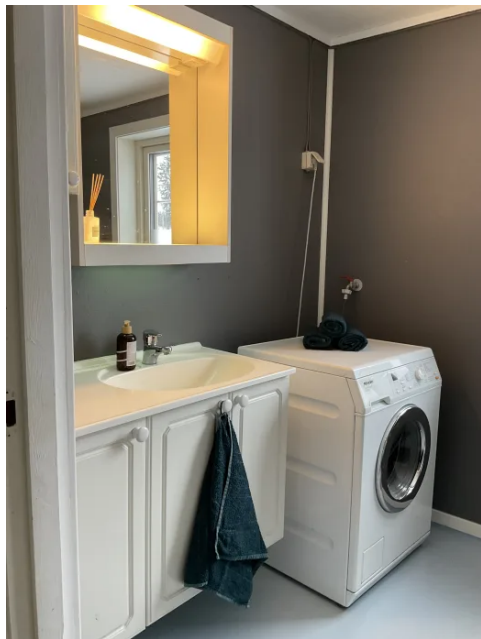
Opplegg for vaskemaskin
