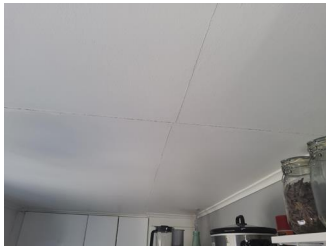
Overflate himling - Sprekker i himling.
