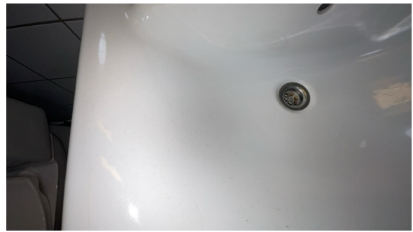
Riss i servant
