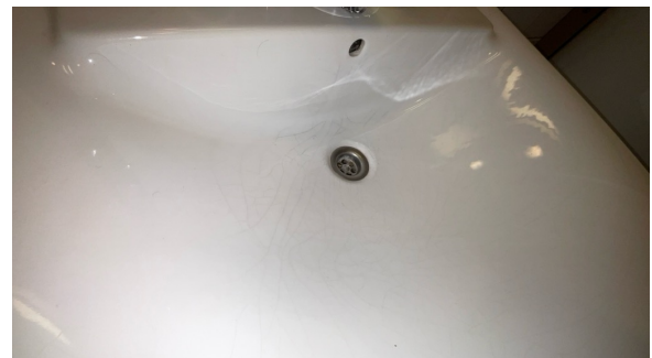
Riss i servant
