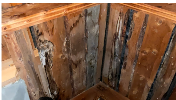
Eldre fuktmerker i himling
