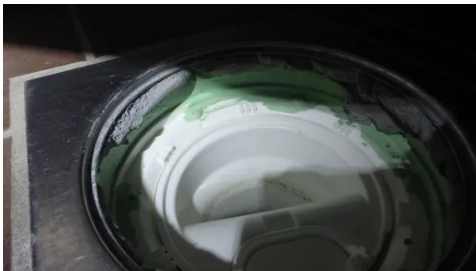
Sluk under servant.
