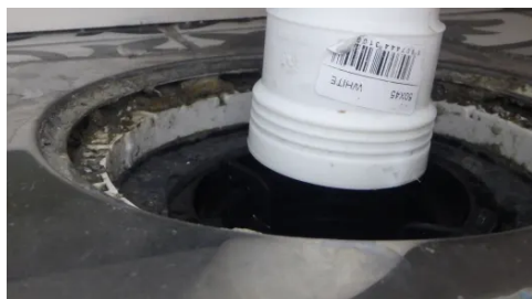
Sluk under benk.
