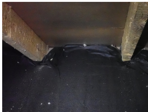
Manglende lufting langs raft
