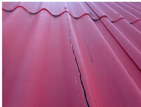
Sprekker i takplater
