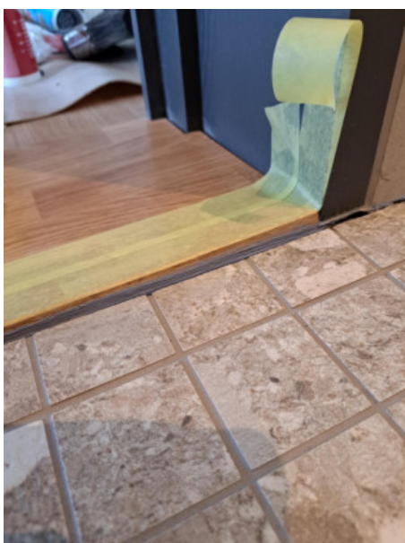
9 (Apartment floor 6, Shower room doorback, 16.03.2025.jpeg)
