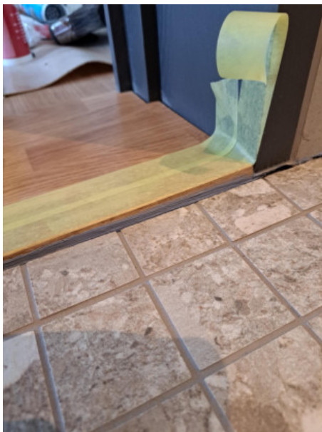
9 (Apartment floor 6, Shower room doorback, 16.03.2025.jpeg)
