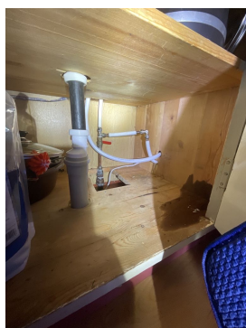
Stoppekran under kjøkkenvask.
