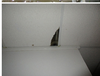
Noe skadet system himling
