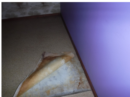
Fukt under filtbelegg
