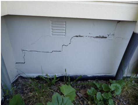
Sprekker i mur under VF
