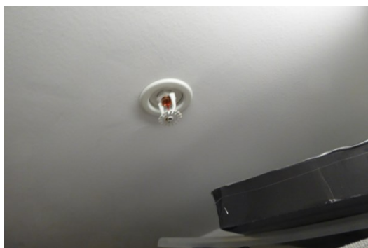
Sprinkelhode i himling.
