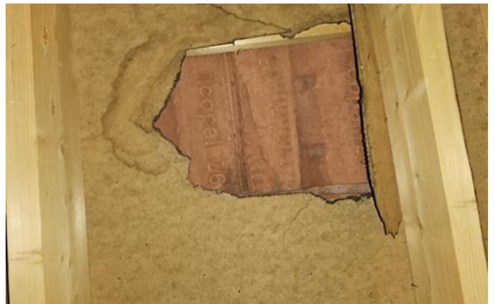
Overflater vegger/undertak - [Hull i undertak.]
