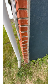
Sprekk i overgang teglstein i front
