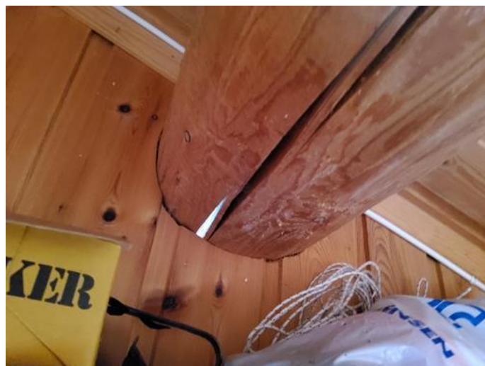
Overflater himling - [Sprekker i drager]
