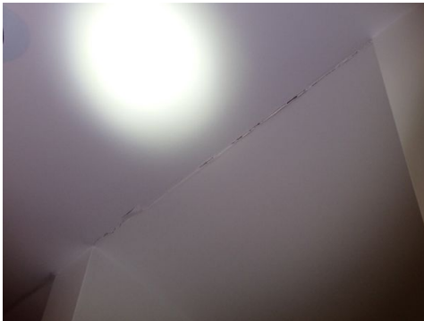
Oppsprekking i himling
