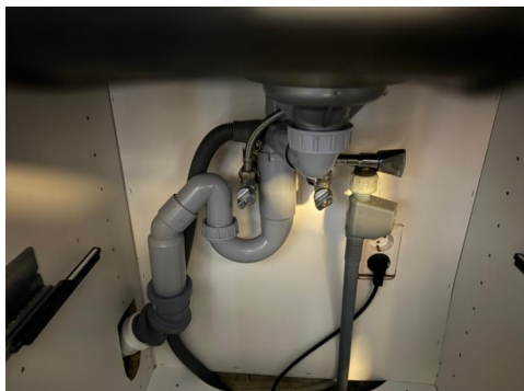
Røropplegg under vask.
