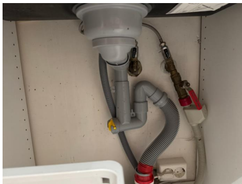
Røropplegg under vask.
