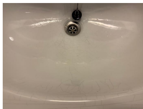
Riss/krakelering i servant.
