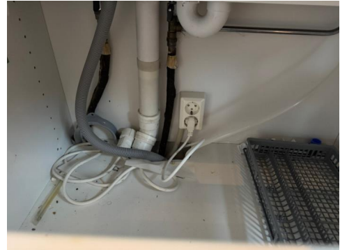
Røropplegg under vask.
