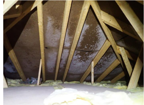
Kondensmerker/mugg i undertak
