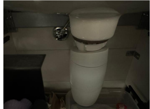
Røropplegg under servant.
