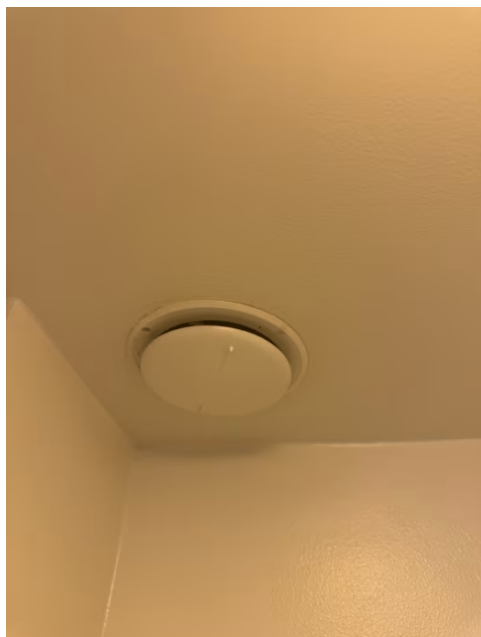
Ventil i himling.
