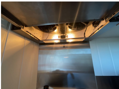
Kjøkkenventilator. Filter mangler.
