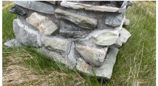
Sprekker i pipe over tak
