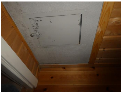
Manglende plate under sotluke
